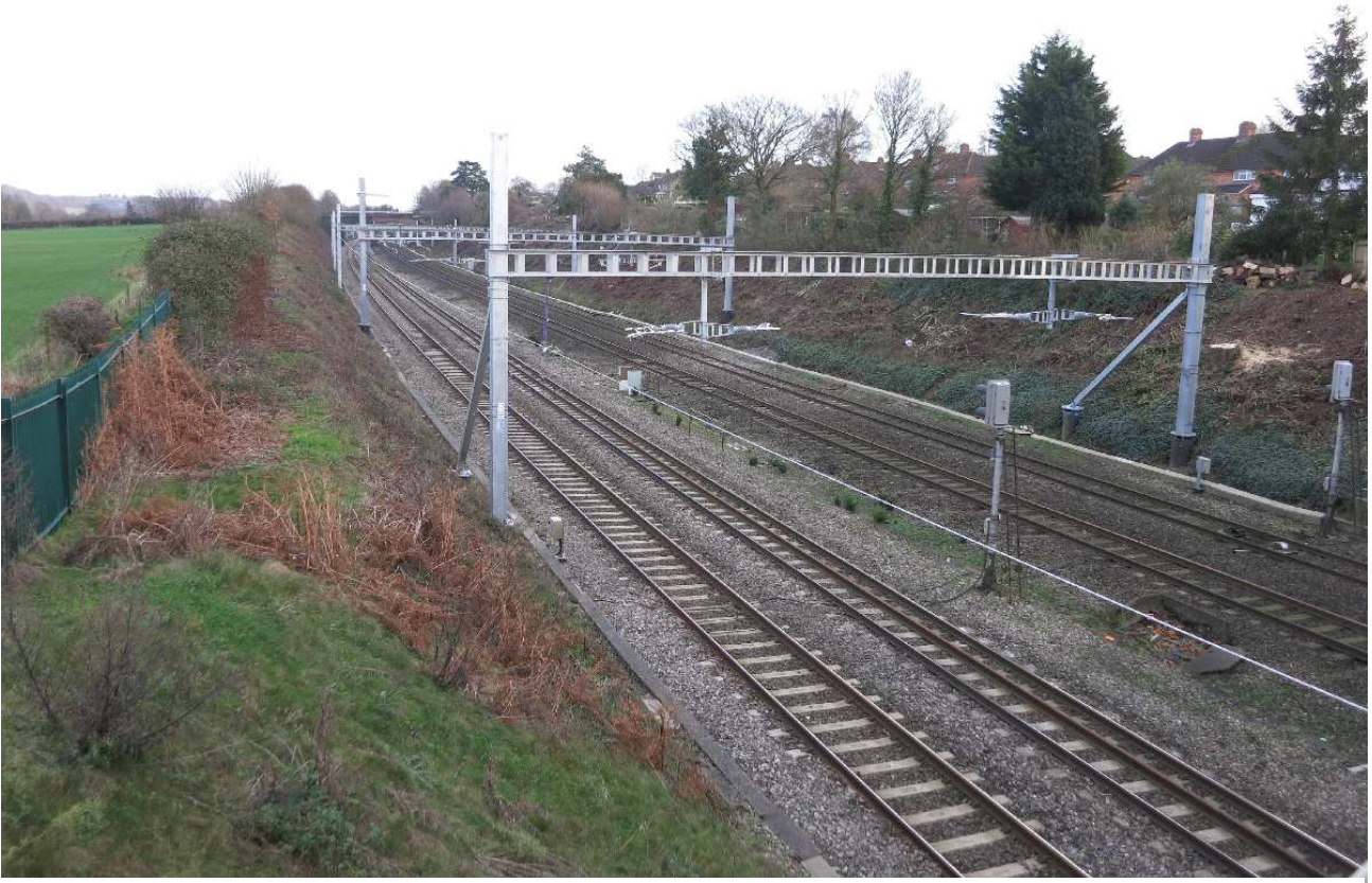
The new grey electrification gantries east of Westbury Lane
